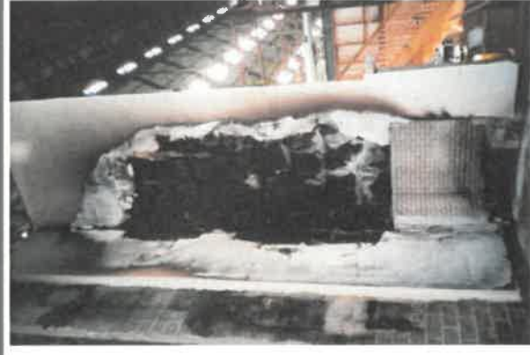
Figure 10: Thermosetting core without adequate fixings or fire breaks
